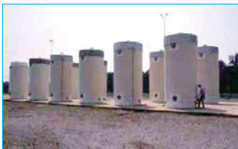
Currently, used fuel is being stored in dry cask storage as well as in the spent fuel pool at Plant Farley. This photo shows an industry dry cask storage site.
