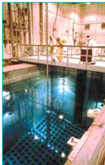
Spent Fuel Pool
