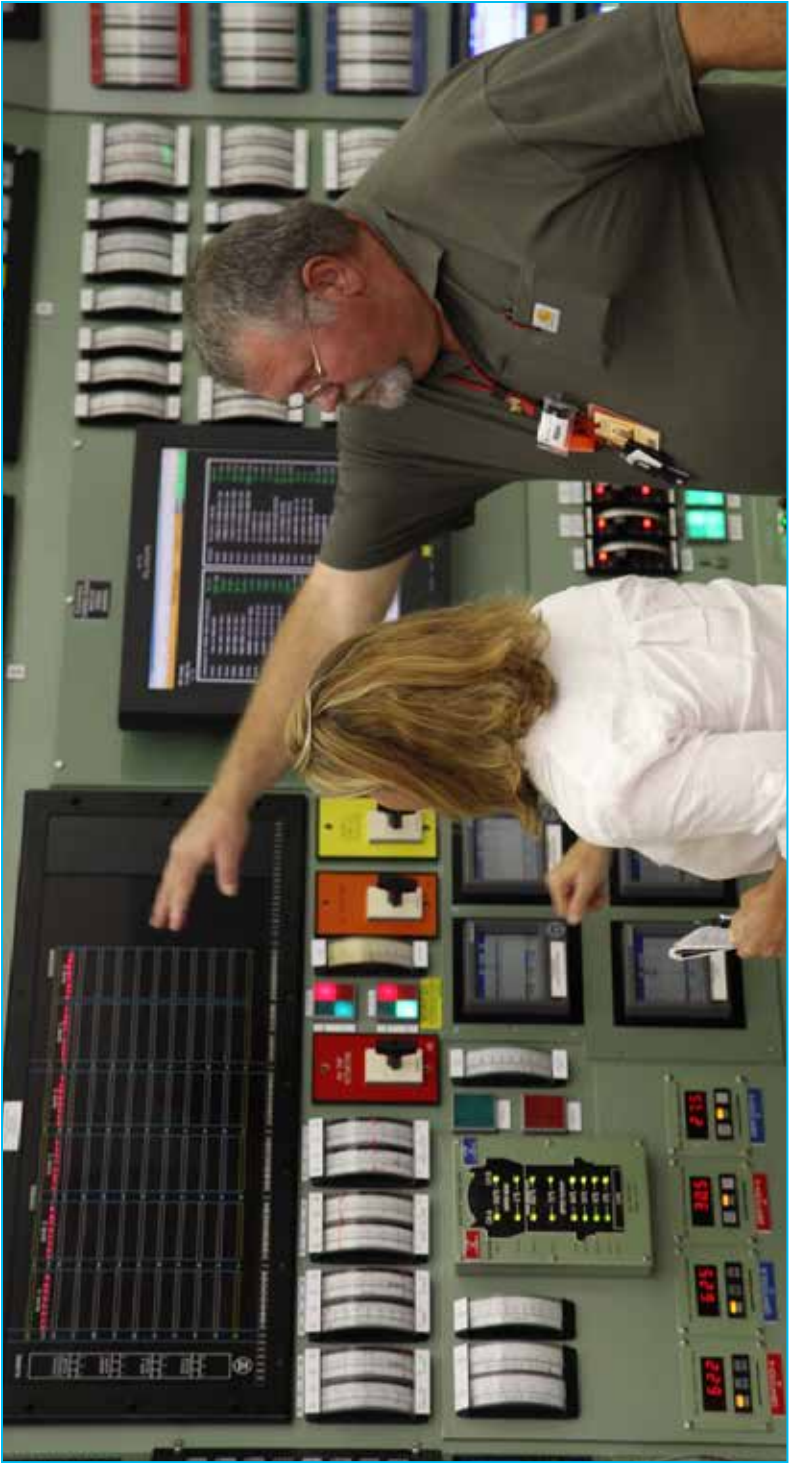
A licensed senior reactor operator explains control room operations to a reporter in the simulator during annual site media day.
