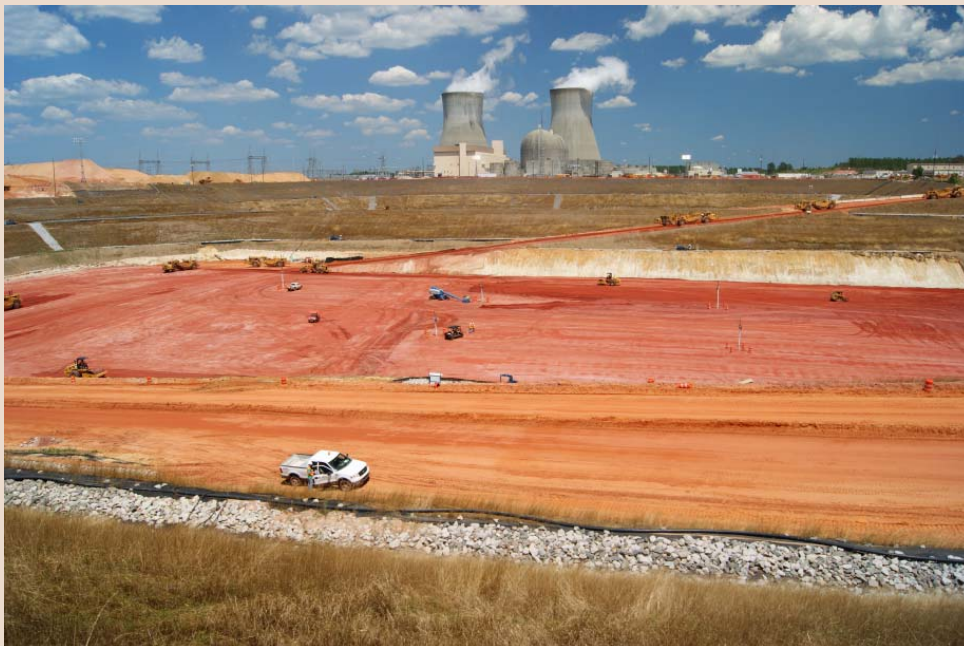
More than a thousand people are currently working at the construction site for Vogtle 3 and 4, with many of them involved in excavating and then backfilling two 90-foot deeps holes in which the new electric generating units will be built. Approximately 900 people also operate and maintain Vogtle 1 and 2, which began generating electricity in 1987 and 1989 respectively.
