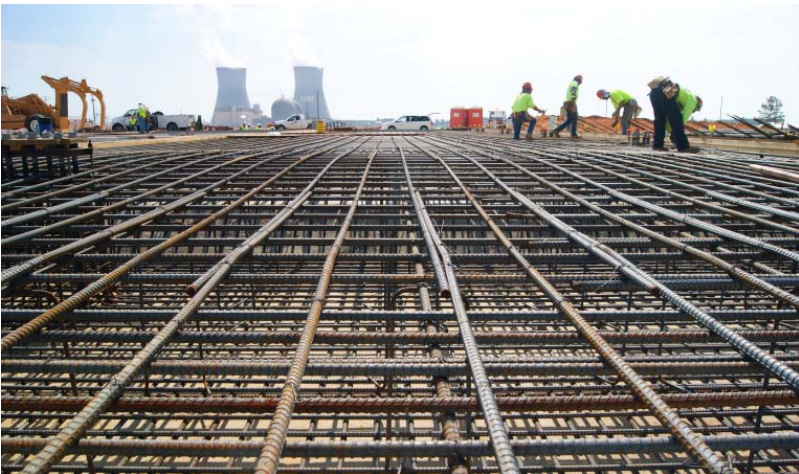
Construction of facilities has begun that will be used to assemble large plant components and modules.
