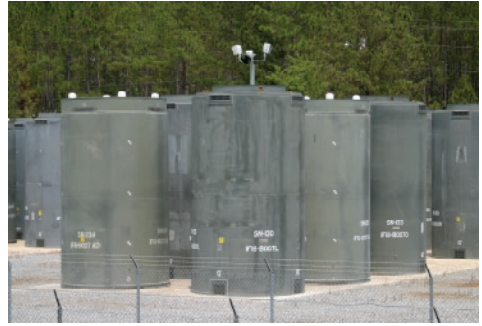
Dry storage at Plant Hatch
