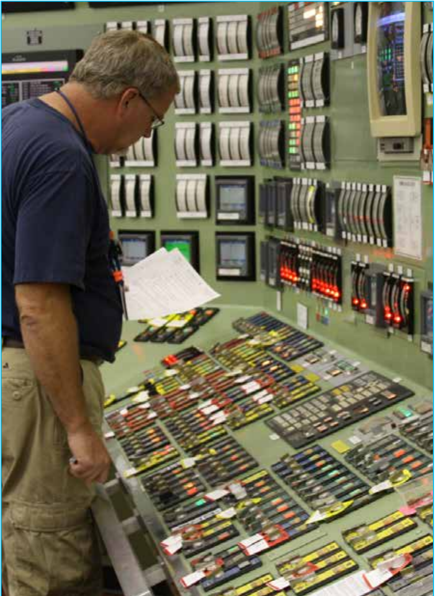
A Plant Operator surveys the board in the Unit 1 Main Control Room during a refueling outage.
