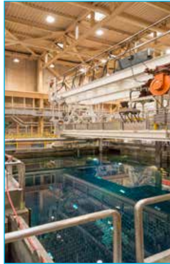
Spent Fuel Pool
