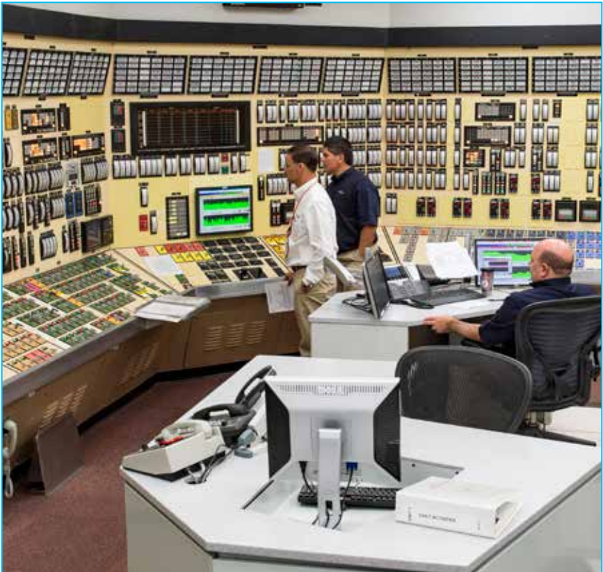
Licensed operators monitor plant operations from the control room of Vogtle Unit 1.
